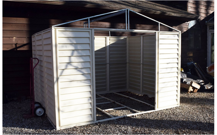
The new shed with the beginnings of the steel roof structure installed. A little ladder work is needed from this point on.
